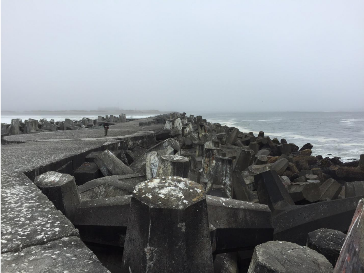
Figure 10: View from the head section of the North Jetty toward the shoreline (August 2016). This area was extensively repaired in the early 1970s. Note the extensive coverage of 42 dolosse and high crest elevation.
